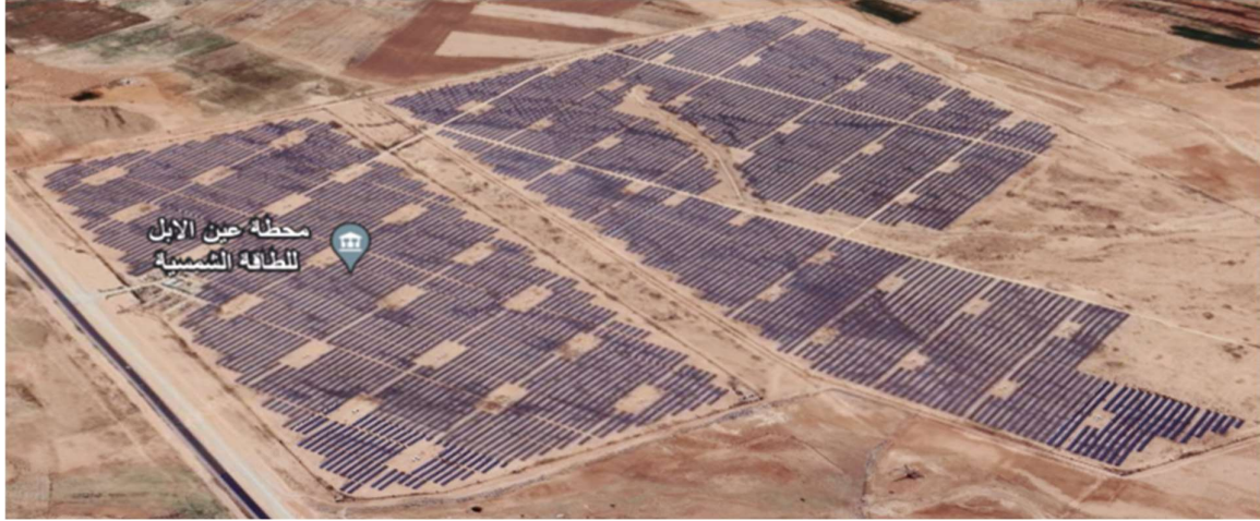
Figure 3: Djelfa solar PV plant [38]
